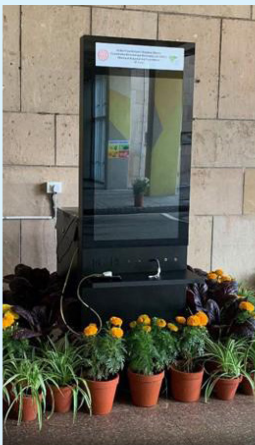
Image: Vanadium Redox Flow Battery installed at IIT Delhi Campus
